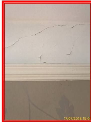
4.4.1 Cracking to plaster above the dado .
