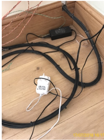
6.12 CCTV kit / router
