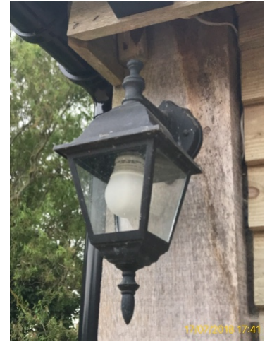
1.5 Lighting (Outside Areas)
