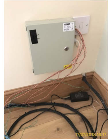
6.12 CCTV kit / router
