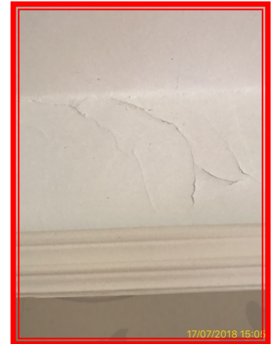
4.4.1 Cracking to plaster above the dado .
