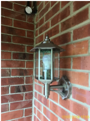
18.6 Lighting (Outside Areas)
