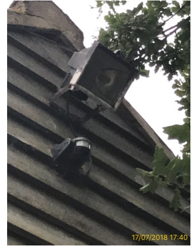
1.5 Lighting (Outside Areas)
