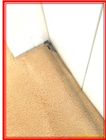
9.6.1 Carpet lifting along on edge of airing cupboard .
