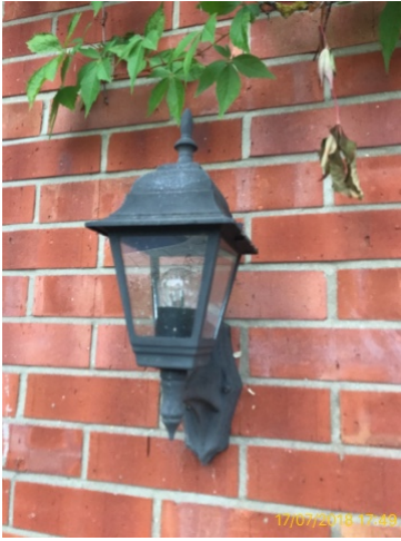
18.6 Lighting (Outside Areas)
