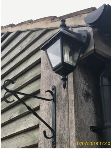
1.5 Lighting (Outside Areas)
