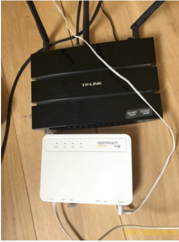
6.12 CCTV kit / router
