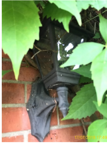
18.6 Lighting (Outside Areas)
