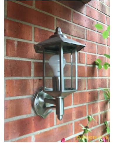
18.6 Lighting (Outside Areas)
