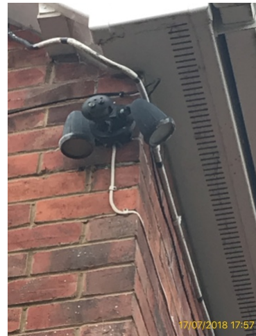
18.6 Lighting (Outside Areas)
