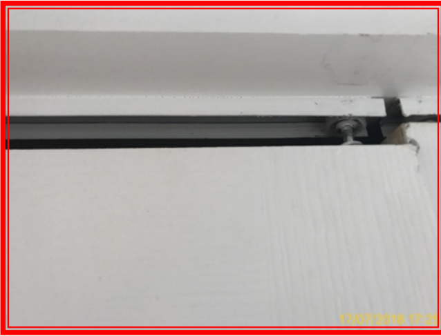
9.3.1 Door on airing cupboard not shutting properly .
